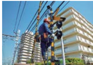
Scheduled inspection of secure communication equipment
